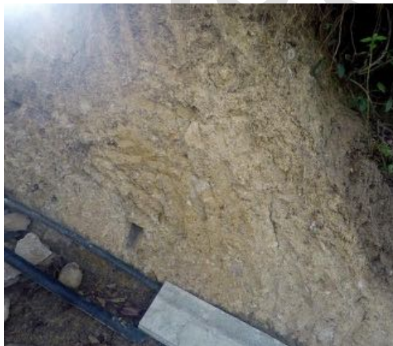
Figure 3.11 Road excavation portraying the lack of bedding and ill-sorted composition of the deposit near its crest. Taken at 15.41°N 121.37°E with a facing direction of N35°E.
