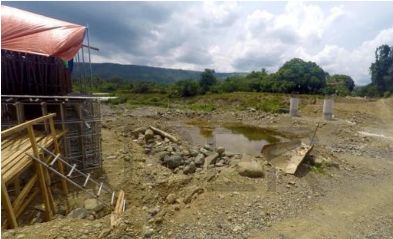
Figure 3.43 View looking S35°W taken at 15.39° N, 121.39° E showing the artificial bed excavation for bank heightening purposes in the Langawan River.
